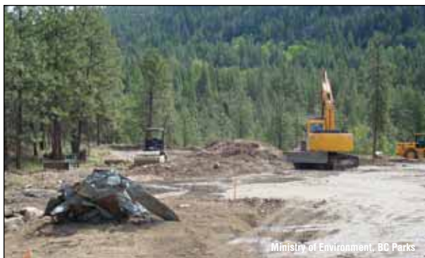
Site disturbance at Skaha Bluffs Provincial Park.
